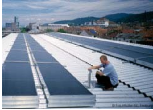
Figure 2: Sorption-assisted air conditioning: collector system on the rooftop of the Chamber of Commerce and Industry in Freiburg, Germany. Photo: Fraunhofer ISE.
